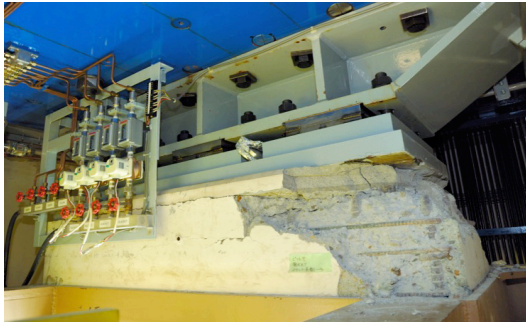
The damage of main props supporting the K=110 MeV cyclotron.
